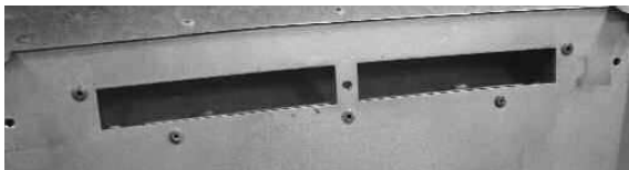
Fig 4 - Flue Restrictor Baffle Not Fitted
